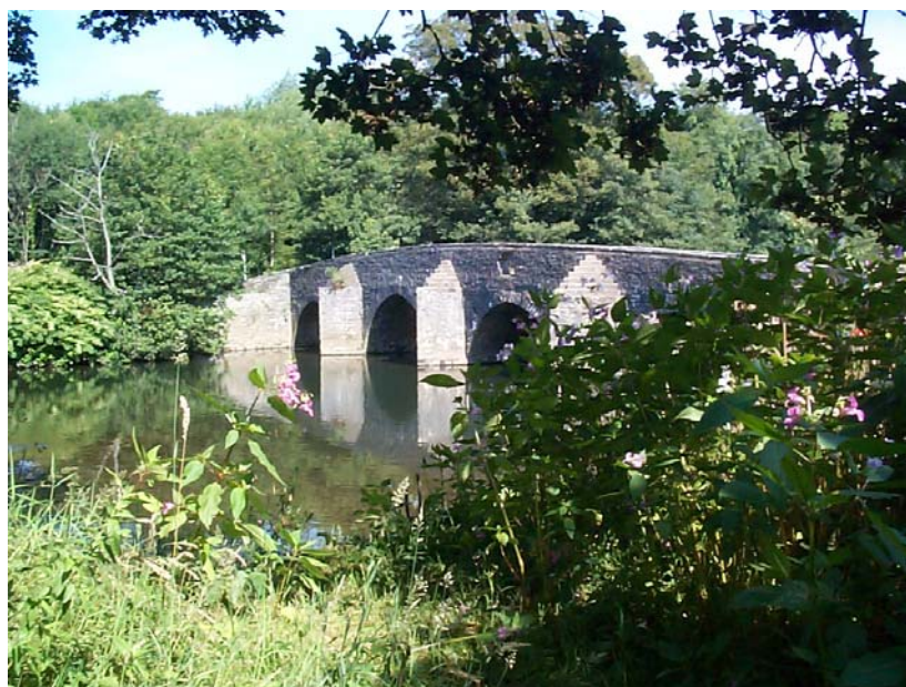
New Inn Bridge (HLCA 016) Merthyr Mawr, Kenfig and Margam Burrows Historic Landscape
